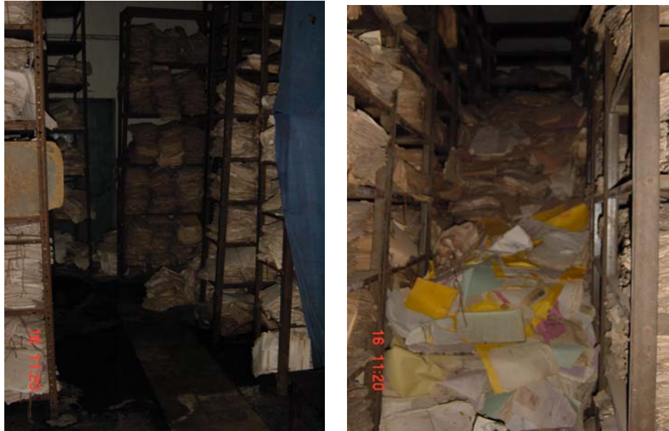
The figure on the left shows the medical records getting damp due to leakages in the ceiling of the record room. The figure on the right shows medical records being dumped in a corner of the room without any classification or proper schedule of destruction. Can anyone retrieve a particular medical record from the dump?
